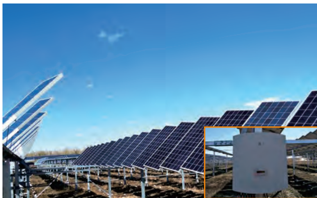
Hebei Zhangbei Agricultural-photovoltaic hybrid PV plant 50MW
