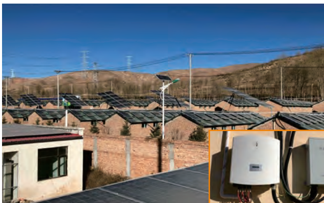
Qinghai HuzhuBanyan poverty alleviation PV Plant 2MW
