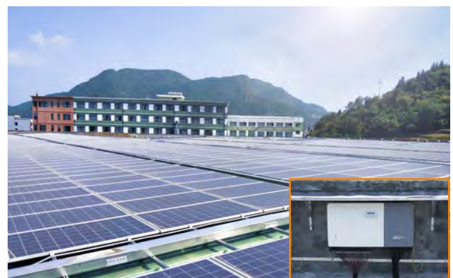
Tyco Electric, Panan Jinhua Zhejiang 1.5MW
