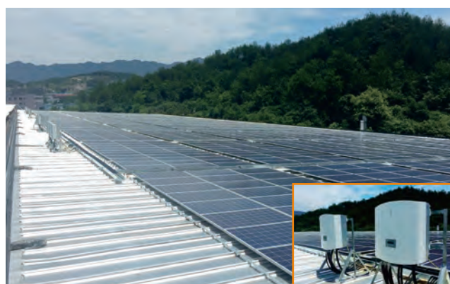
Hainan JiuLongGlass 1.7MW
