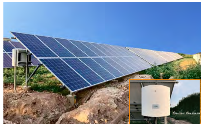
Hebei Qinghuangdao poverty alleviation PV Plant 5MW
