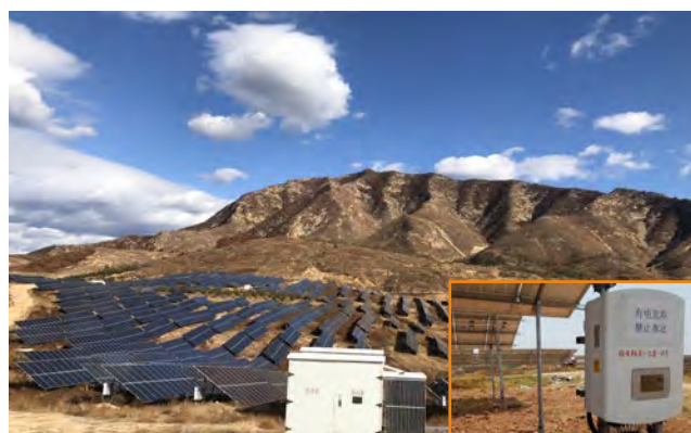
Liaoning Gaizhou Jiuzhai PV plant 20MW
