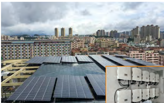
Shenzhen Jiangnan Times Building 600kW
