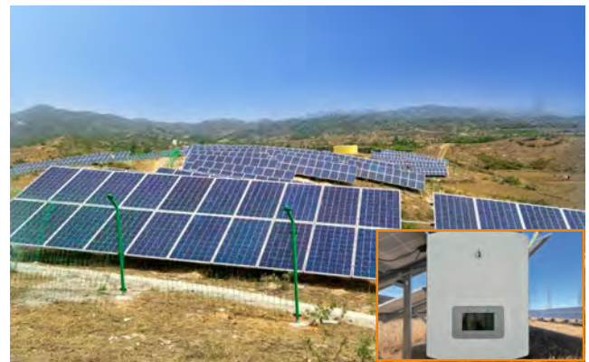
Hebei Qinghuangdao poverty alleviation PV Plant 9.7MW
