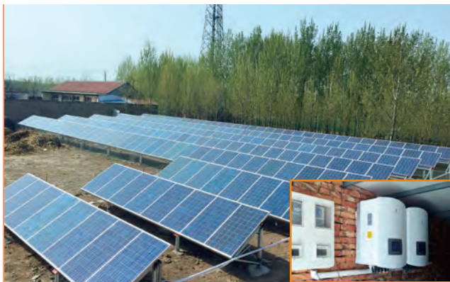
Shandong Leling poverty alleviation PV Plant 50kW
