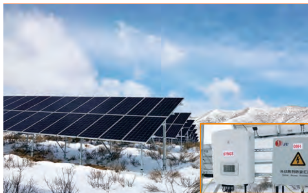
Shanxi Guangling PV plant 1.47MW
