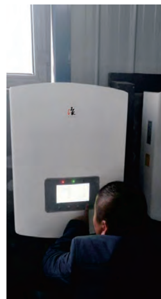
Heilongjiang PV plant
