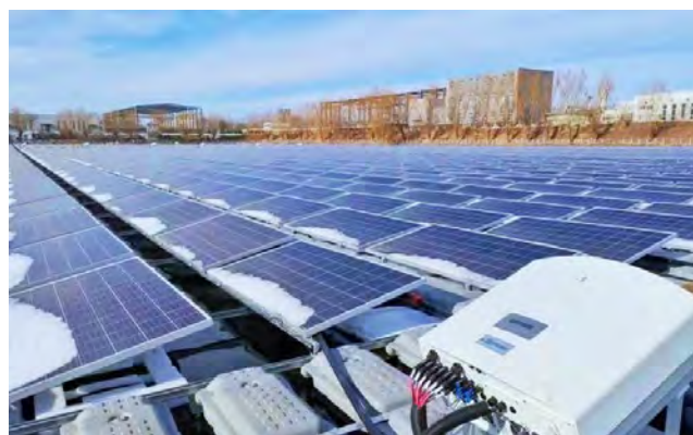
Beijing Shunzhen Green Harbor's Plant 5.5MW
