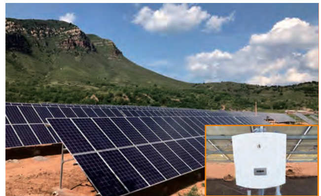
Shanxi Xiyang poverty alleviation PV Plant 7.2MW
