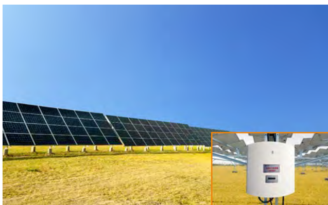
Huaneng Yimin surface mine PV plant 20MW
